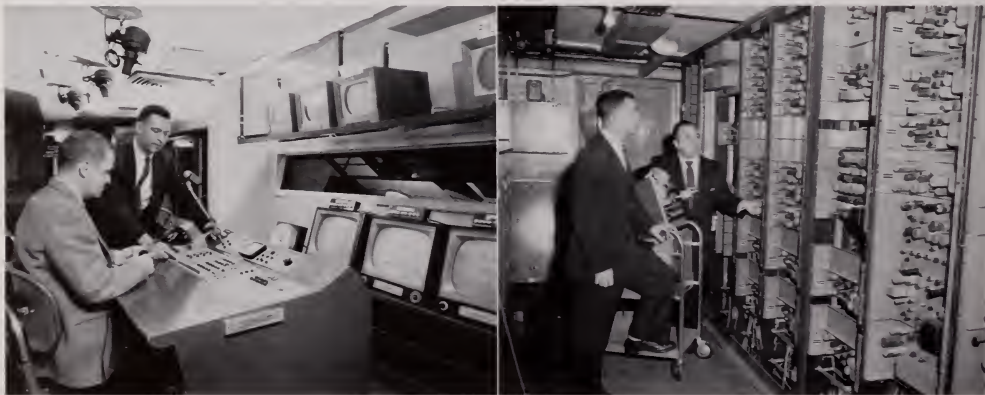
(Left photo) In the 6B control room, project engineer Jerry Rester (standing) explains the functioning of the new panel to technical director Noel Warwick. (Right photo) In the equipment room on the fifth floor studio section of the RCA Bldg., where Rester (left) looks on as Ed Pores, the engineer who conceived the video new system for 6B, tests the equipment.
